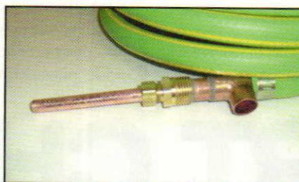
The copper tee fitting slides over the 3/8” copper tubing of the chiller.
