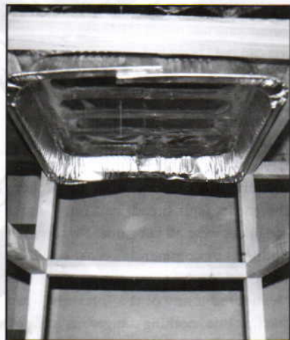
FOIL HOOD FOR BOILER
